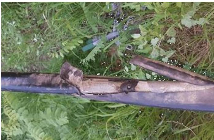
Figure 4: Damaged cable insulation.
