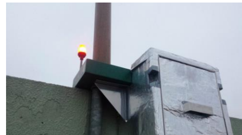
Fig. 2. Current sensors installed on the lightning rods of buildings P1 and P2 (upper picture) and detail of the installation (lower picture).
